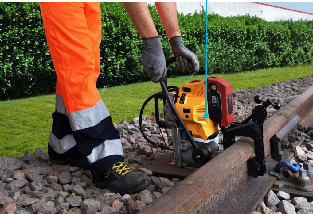
Sleeper drilling machine
