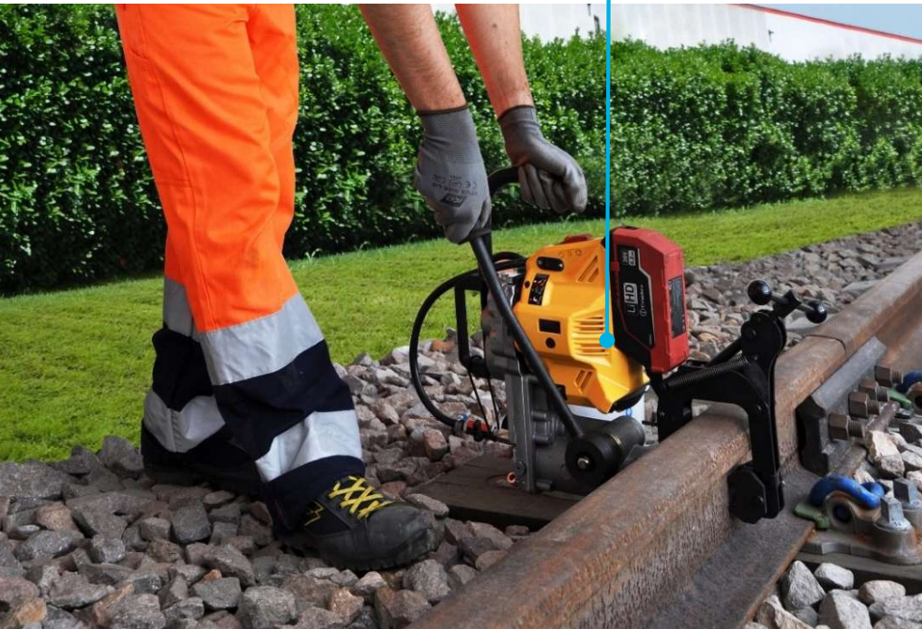
Sleeper drilling machine
