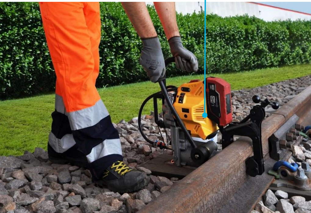
Sleeper drilling machine
